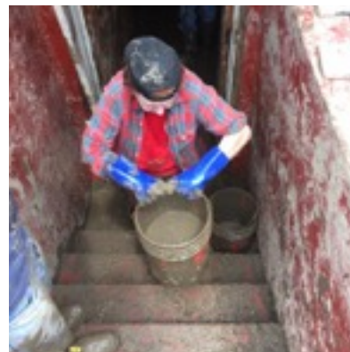
A volunteer helps clean mud and debris out of a Marshall County home damaged during the July 2017 flood that swept through northern West Virginia.
