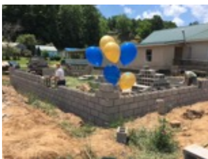
Volunteers lay the foundation for a new home in a Clendenin neighborhood that was damaged during the June 2016 flood.
