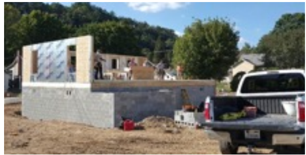
Volunteers work on a rebuild in Greenbrier County after the June 2016 flood.
