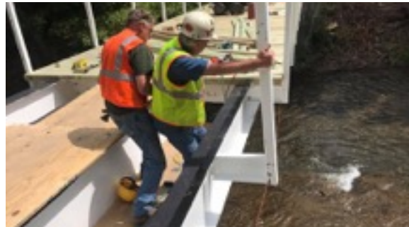
The new Elmer Brown Bridge in Mingo County gave 12 families access to their homes after a bridge was destroyed in a 2015 flood.
