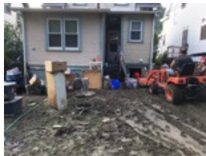
Member agencies spent time doing site cleanup after the July 2017 flood so that home repairs and reconstruction could begin.
